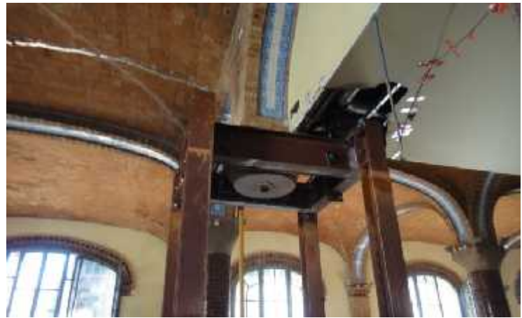
Photo 3. Column eliminated. Optical fiber in vault.
