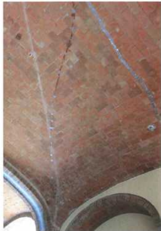
Photo 1. Optical fiber in vault.
